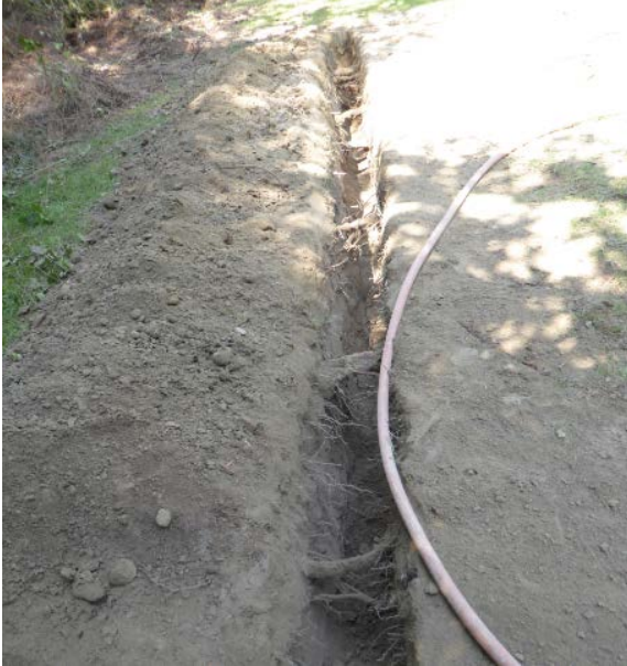
Photo 2. View looking to the north along the east trench. This view shows the low density of structural roots encountered.
